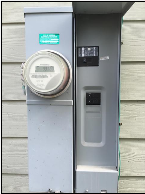
7.6 Item 1(Picture) Main disconnect: Right side
